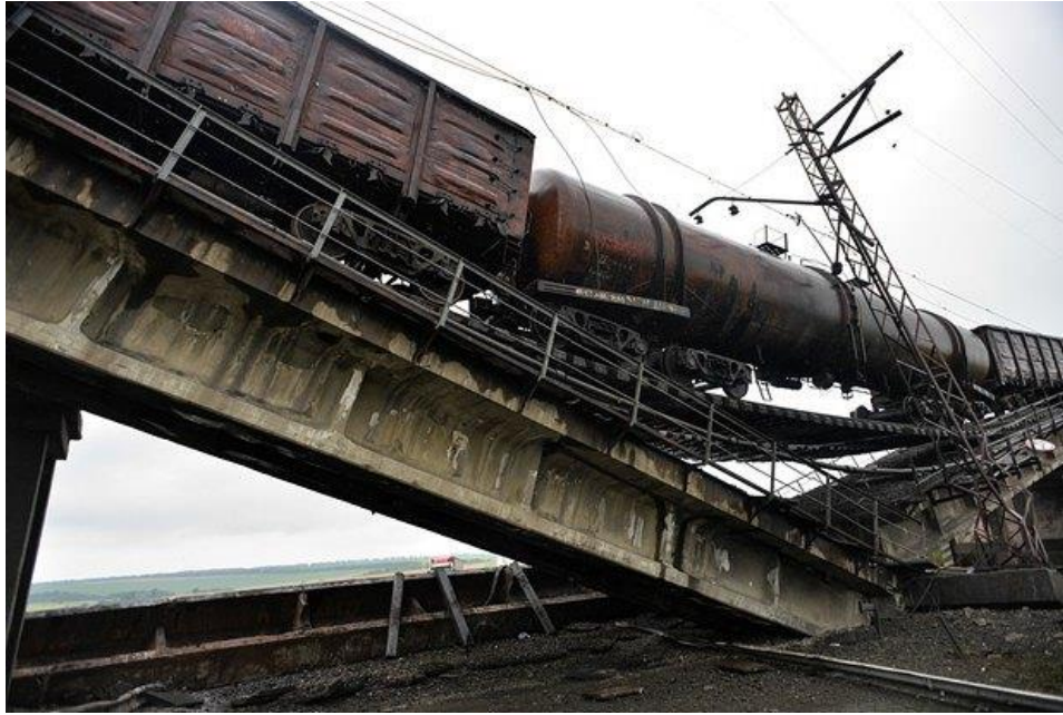
Fig. 4. Destroyed railway bridge.
