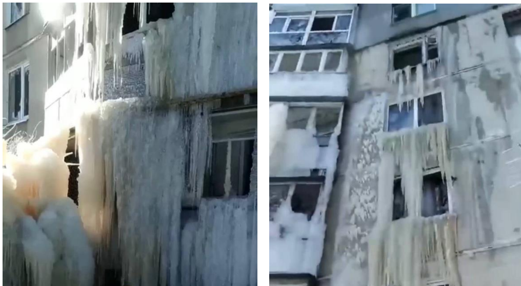
Fig. 1. Heating system violation.
